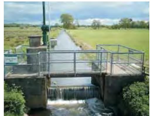
Low power, remote river level monitoring
